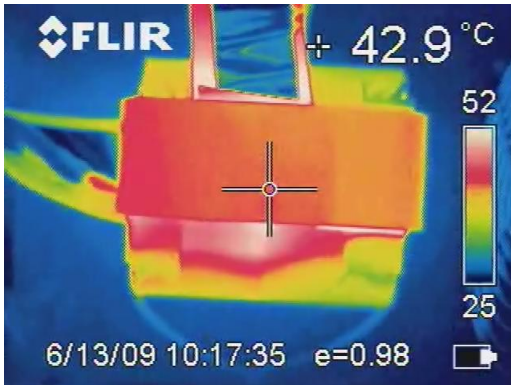
Figure 75 Thermal picture of open air cooled 32 uH inductor at 10 kW
