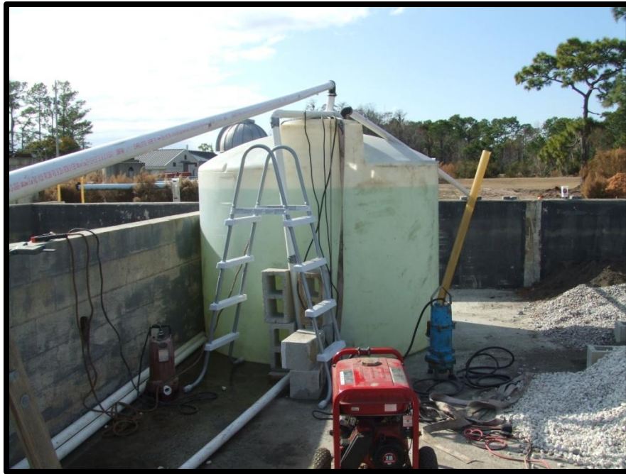
Figure 23: 1,500 Gallon Source Water Tank
