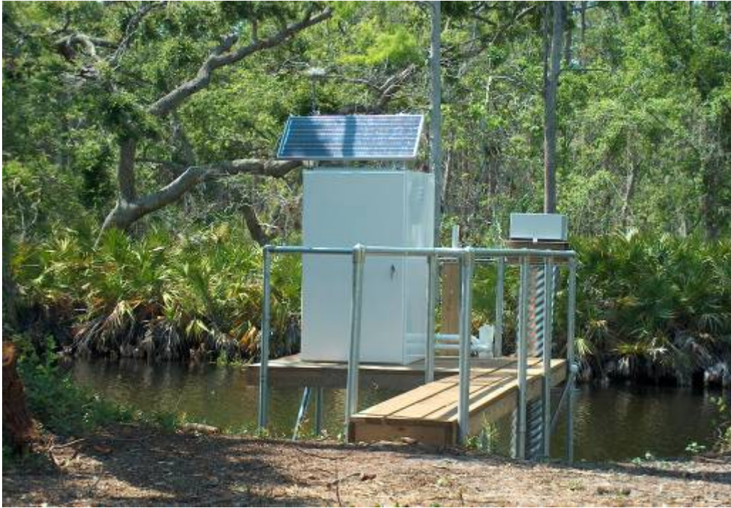
Figure 8: Catwalk Monitoring Station
