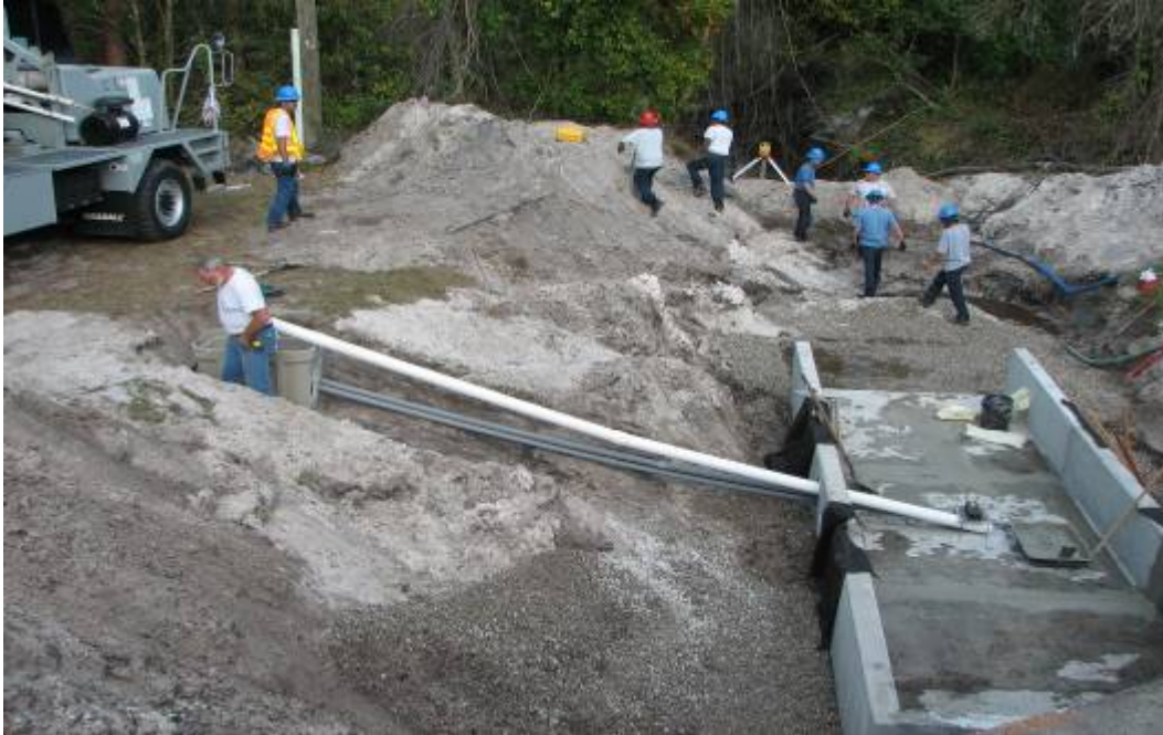
Figure 11: Suppressed Concrete Channel
