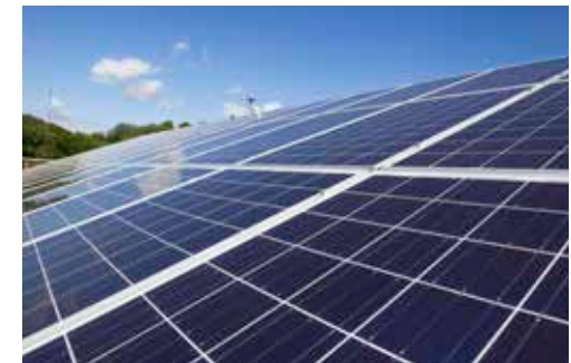
Solar Panels developed by Neelkanth Dhere, a professor at UCF's Florida Solar Energy Center, and his team of graduate students are safer, more efficient and less expensive.
