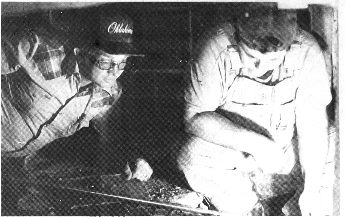
THESE TWO MEN, Glen Pope (left) and Melvin Lancaster, of the maintenance department at Southwestern Oklahoma State University recently completed a big task which solved a 40-year problem in the women's basement restroom in the Administration Building on the Southwestern campus. It seems that since 1941 there have been problems with backed up sewers in the restroom, so it was decided this year to look into the problem and see what was actually wrong. Pope and Lancaster spent many hard and long hours in close, cramped quarters to dig up the pipes to find the problem. It seems that when the building was built, concrete was poured into the plumbing which has caused problems for more than forty years. Thanks to Pope and Lancaster, the problem is now solved.
