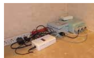
Development of H 2 S monitoring system
