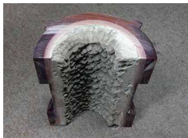
Fig.2 Pipe with Talc scale 3 month elapsed.
