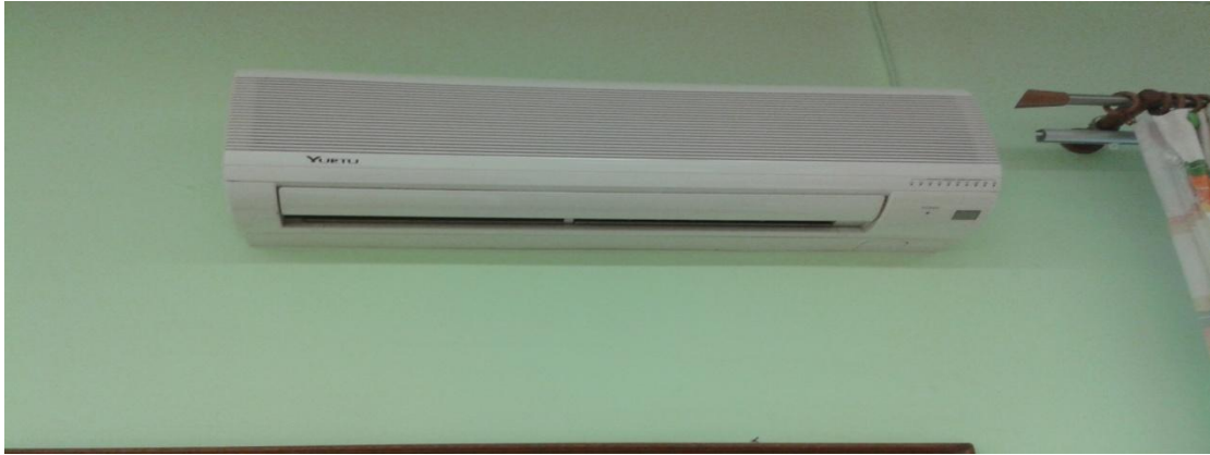
Figures 26: Two types of installed air conditioners
