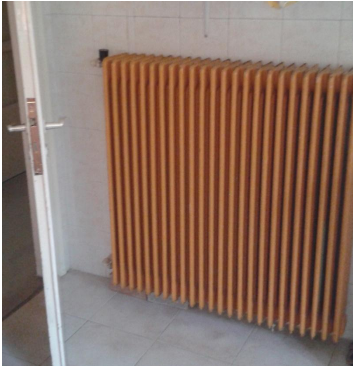
Figure 26: Photograph of a typical radiator in a bathroom. These comprise of the emission system of the heating system.
