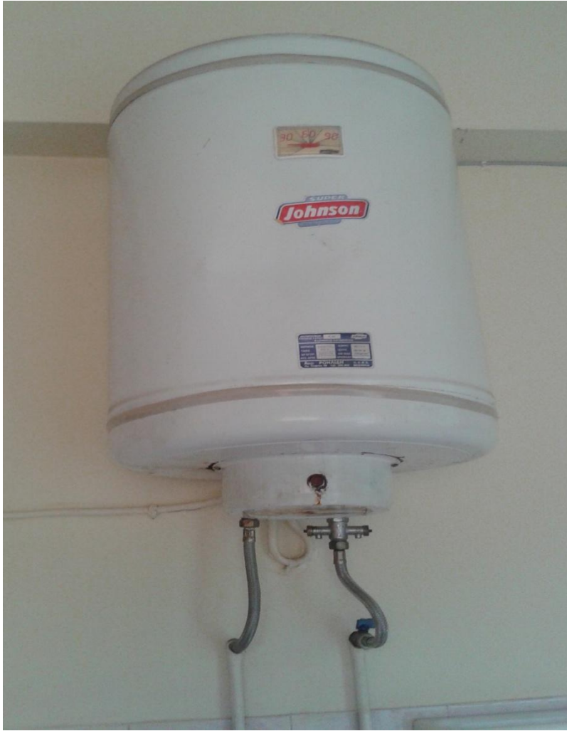
Figure 27: Electrical water heater boiler
