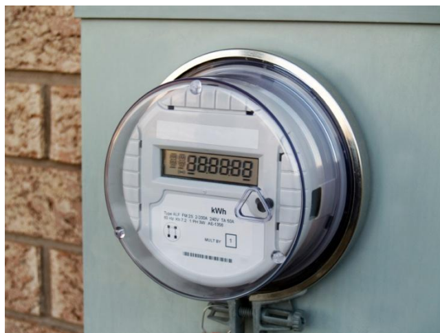
Figure 6 - Smart Electricity meter
