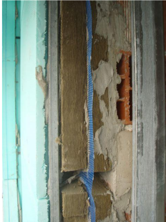
Picture 68: External insulation of the studio-apartment; from left to right, 5 cm of extruded polystyrene plates, 10 cm of stone-wool and ceramic bricks
