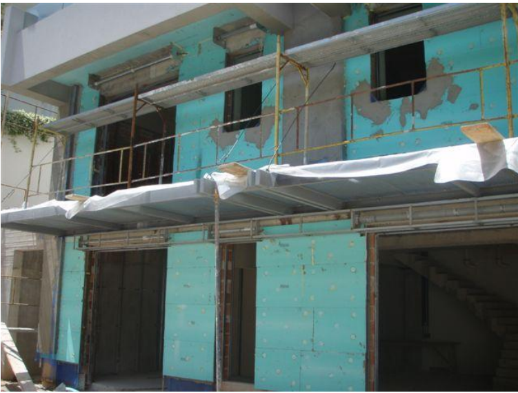
Picture 63: Installation of extruded polystyrene plates in the outer cell during construction
