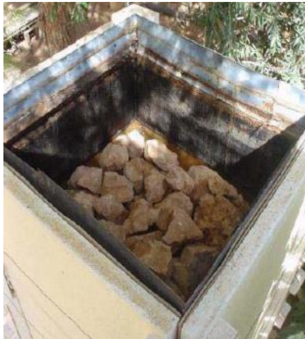
Picture 12: Photo of the Evapo-reflective roof without the aluminum cover
