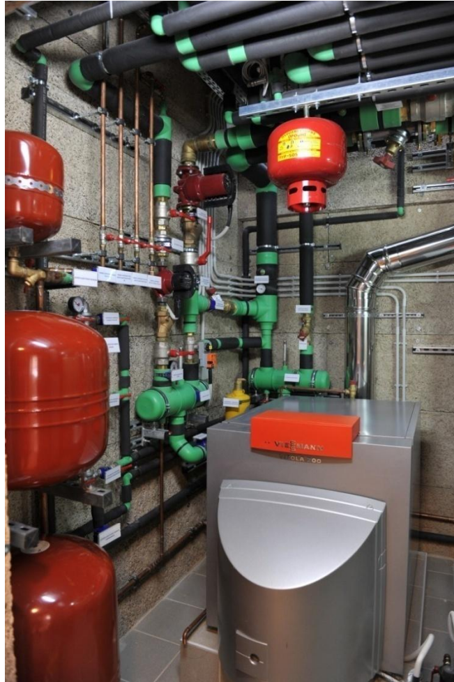
Picture 72: Oil fired boiler Vitola 200 and part of the heating grid. Notice how the pipes use extra insulation to minimize heat losses during the heating medium transfer
