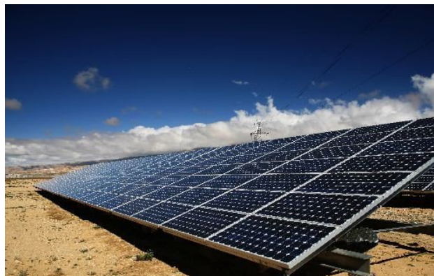
Picture 20: Commercial Photovoltaic Station with one-axis tracking system.
