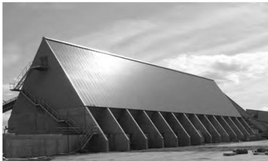
Figure 6: Example of an A-frame flat storage (Obernberger & Thek 2010)
