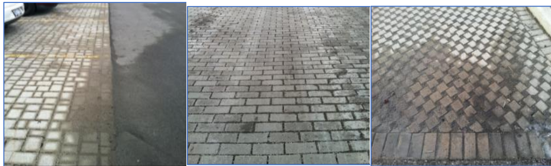
(a) Low severity clogging b) Medium severity clogging (c) High severity clogging
