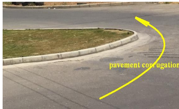
Figure (9) Pavement corrugation around the divisional island
