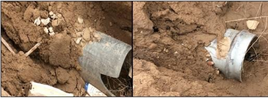
Figure (4) Buried pipes in the study area
