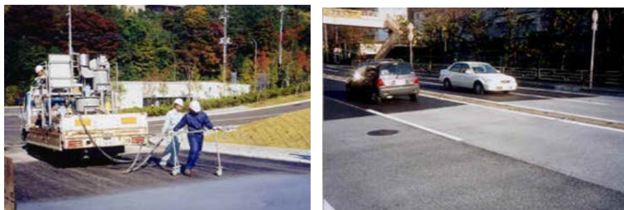
Figure 1-3. The usage of photocatalyst painting on the road to eliminate \text{NO}_x toxic gas from the vehicles in Japan.
