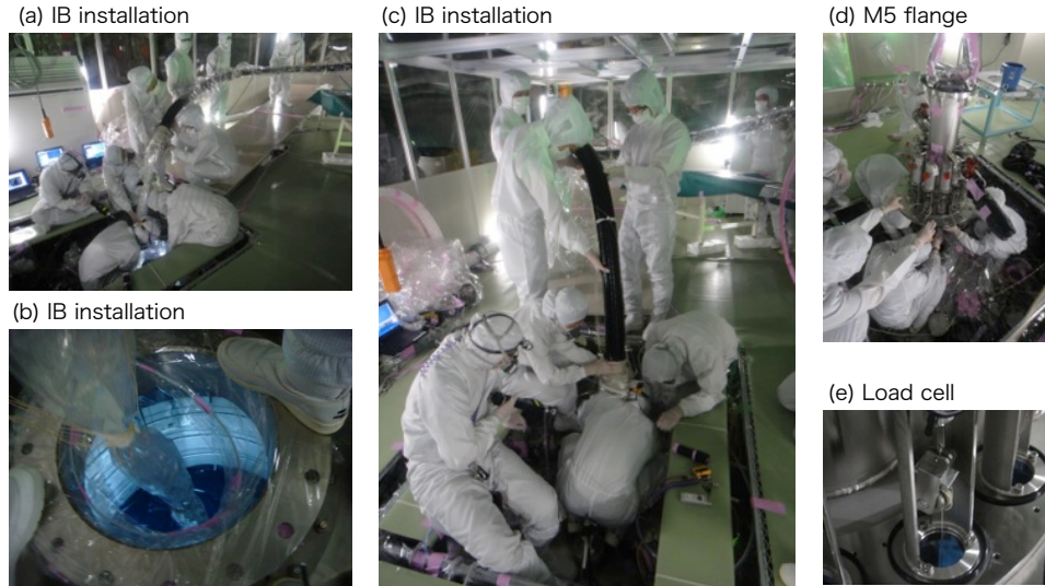
Fig 3.25: Pictures of IB installation. (a)-(c) show pictures during IB manual installation work. (d) shows M5 flange, and (e) is load cell unit attached to the flange to measure the load of 12 strings hanging the IB.
