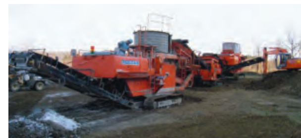
Soil modification using two mobile modification machines. Waste gypsum powder is added to soil in first machine and lime is added in second machine.
