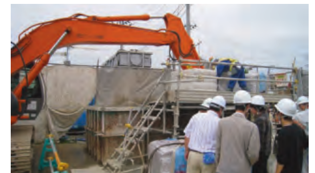
Visit to a site of tunnel excavation for the Sendai city subway(Yakushi-do area) : At this area, the sludge discharged during the ground modification is recycled by the fiber-cement-stabilized method. All of the modified soil is used as road embankment material at Akiu area.
