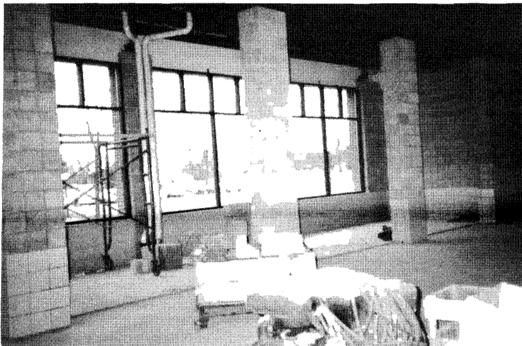
The new student center under construction provides new southern exposure. Construction for phase I started early May of 1994.
