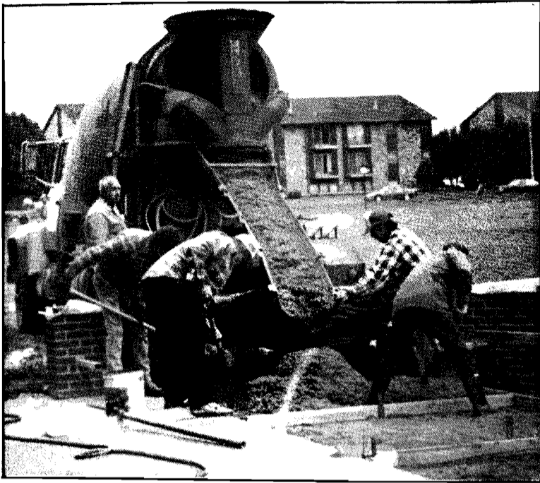
Morty Poling, Don Porter, Paul Miller (supervisor), Judd Rickert, and an unidentified man pouring cement for the new patio.
