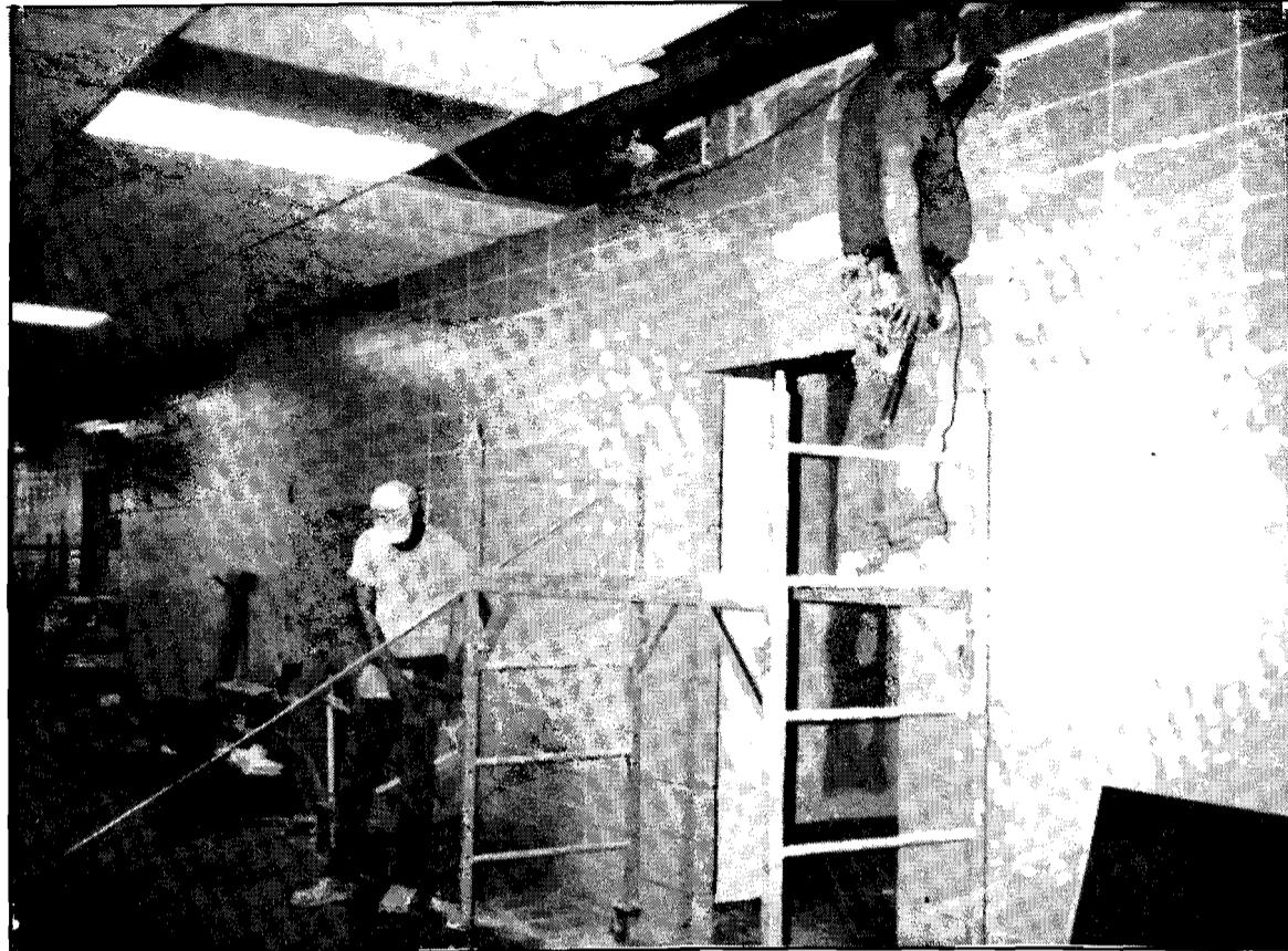
Here are Mike Sharp and Paul Zenor, from H&H of Ames, working on the restroom remodeling project, Sept. 5. The two are employed as drywallers. (Photo by Shannon Hayes)
