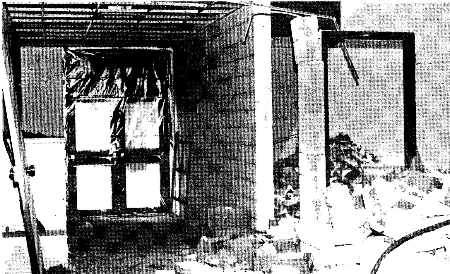
This is the scene beyond the double doors near the main entrance, since the remodeling work began recently. Major work such as demolition of walls and floor leveling is being done near
