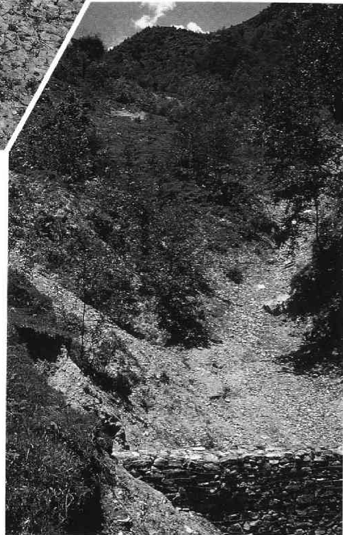
Photo 10 Shallow slides and a gabion-type check dam in a deep-seated slide zone at Kuhire Kateri Samsire, north of Kusma. (Photo by T. Tamura ; May, 1994)
