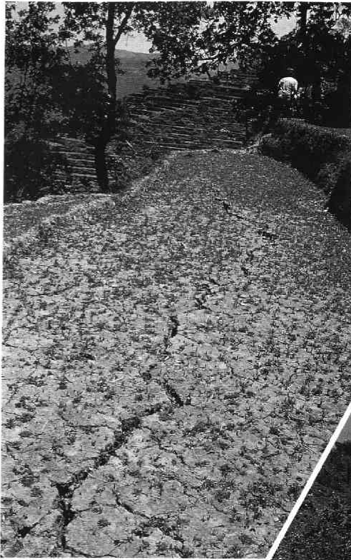
Photo 9 Cracks on abandoned paddy terraces in a deep-seated slide zone at Kuhire Kateri Samsire, north of Kusma. (Photo by T. Tamura ; May, 1994)
