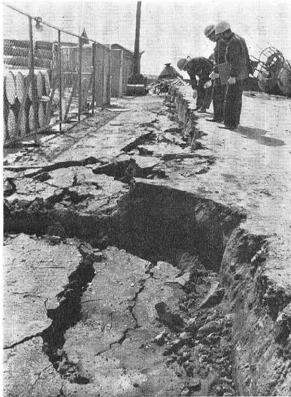
Photo. 12 Fissured yard, Mitsubishi Petroleum Co., Hakodate City
