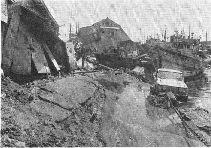
Photo. 13 Subsided Wharf in Hakodate City
