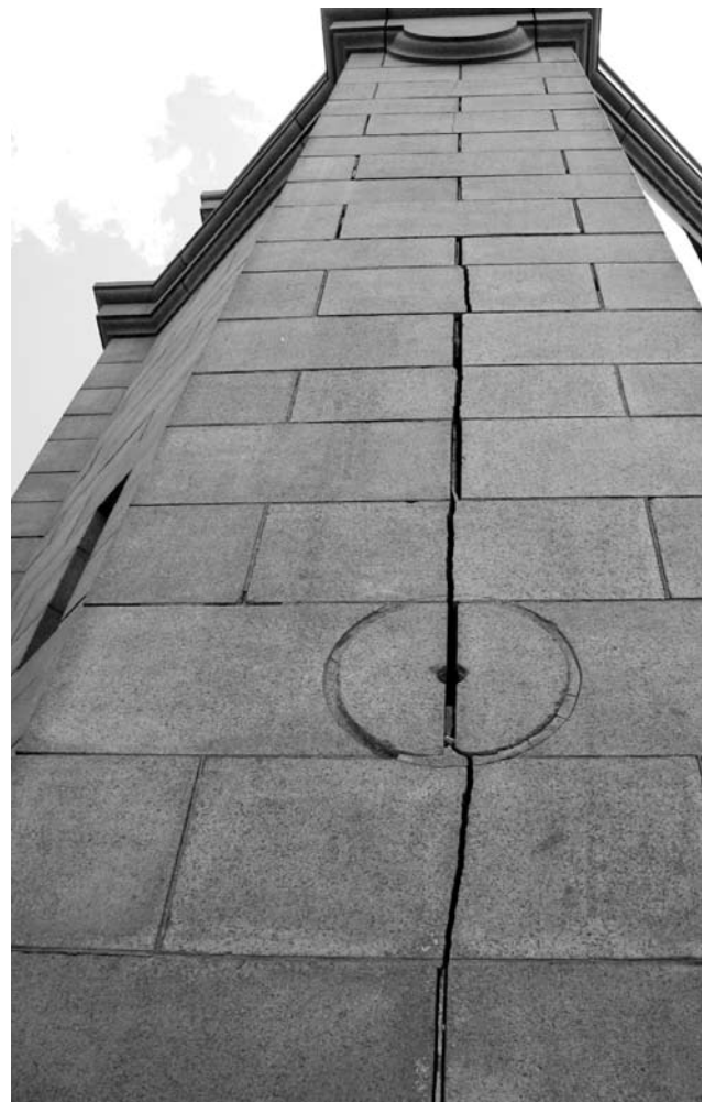
Figure 8: Cracking in Pier (Photo by Peter Begley)
