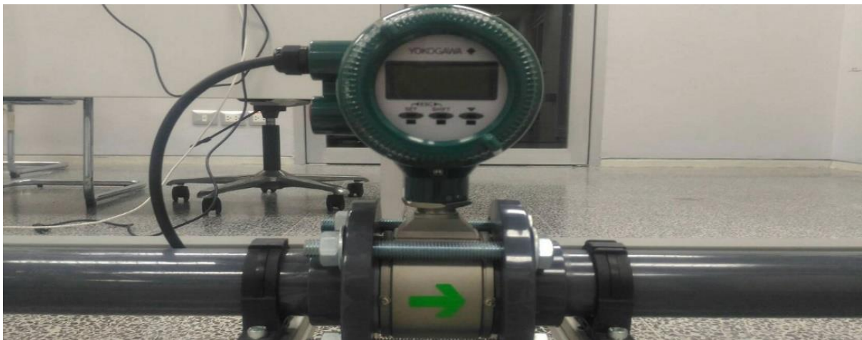
Fig. 5. The standard electromagnetic flowmeter.
