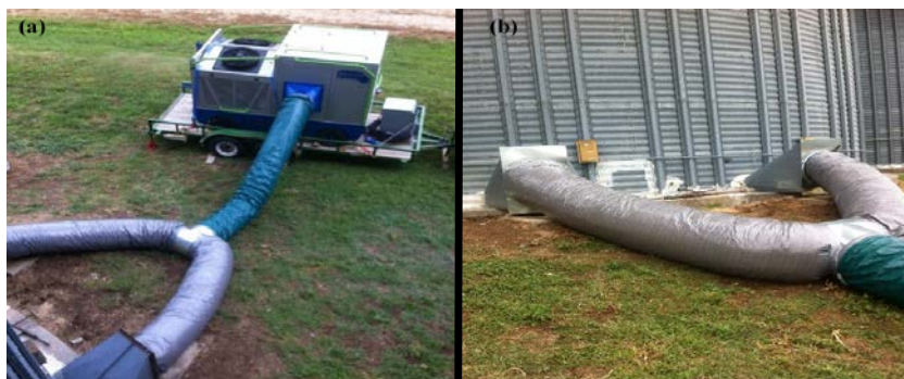
Figure 7. Grain chiller GCH-20 setup: (a) Insulated duct connected to the chiller's outlet at one end and to a "T" connector at the other, (b) Two ducts attached to the fan transition parts of the aeration fans that were removed.
