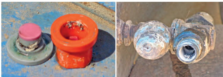
Fig. 6. Bad nozzle condition.
