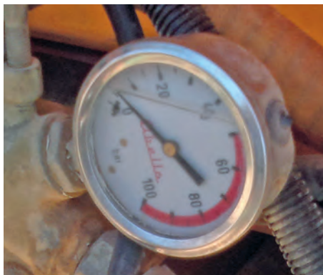
Fig. 5. Inadequate manometer (Excessive scale and insufficient resolution).
