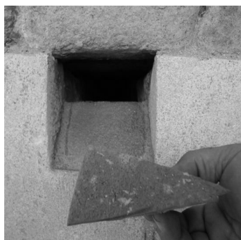
Fig. 1 A scaffold hole modified to be inaccessible for pigeons and allow swifts and bat enter; a wedged piece of brick is shown before the use in the hole
