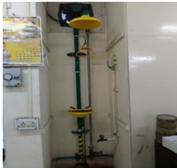
4. Eye wash station
