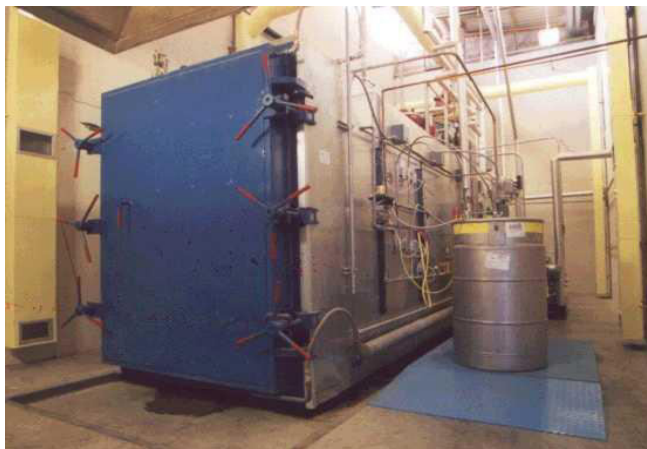
Figure 15: Ethylene Oxide (ETO) sterilization plant.
