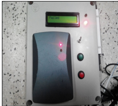
Figure 7: Security box failed condition
