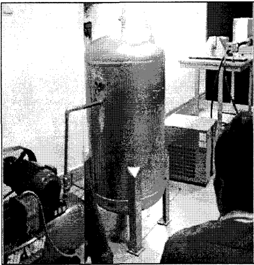
Figure 5: Completed small CAES system
