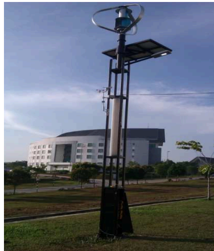
Fig. 1. Hybrid PV-wind System installed at FKE
