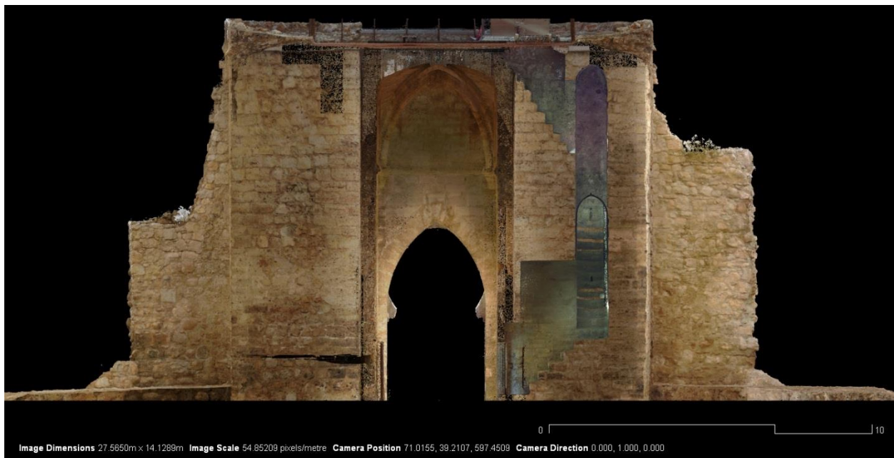
Figure 4 Orthographic image of a point cloud viewing the South elevation with the inside of the gate visible, including the stairwell and arches of the Toledo Gate in Ciudad Real, La Mancha, Spain. Photo: University of South Florida’s Center for Virtualization and Applied Spatial Technologies.
