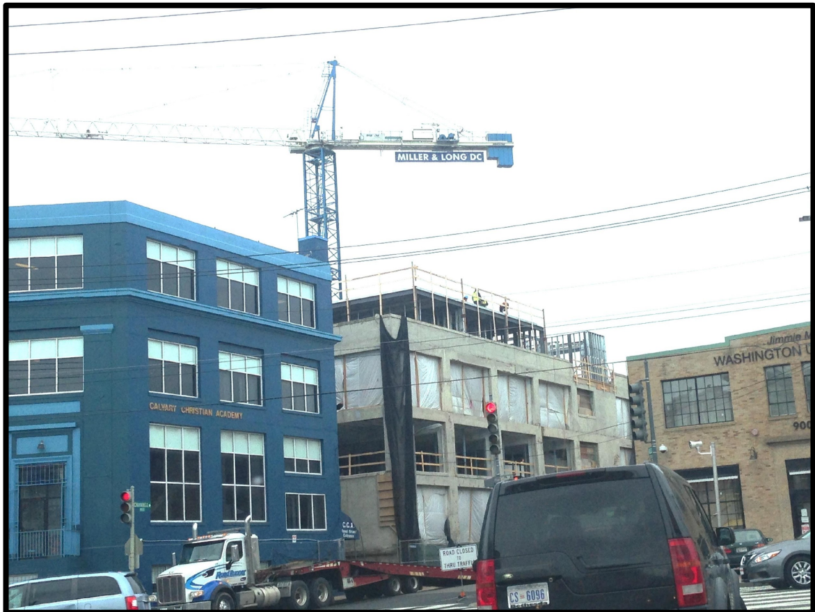
Figure 3. Construction of Evarts building project seen from Rhode Island Ave. Photo taken by author, 2017.
