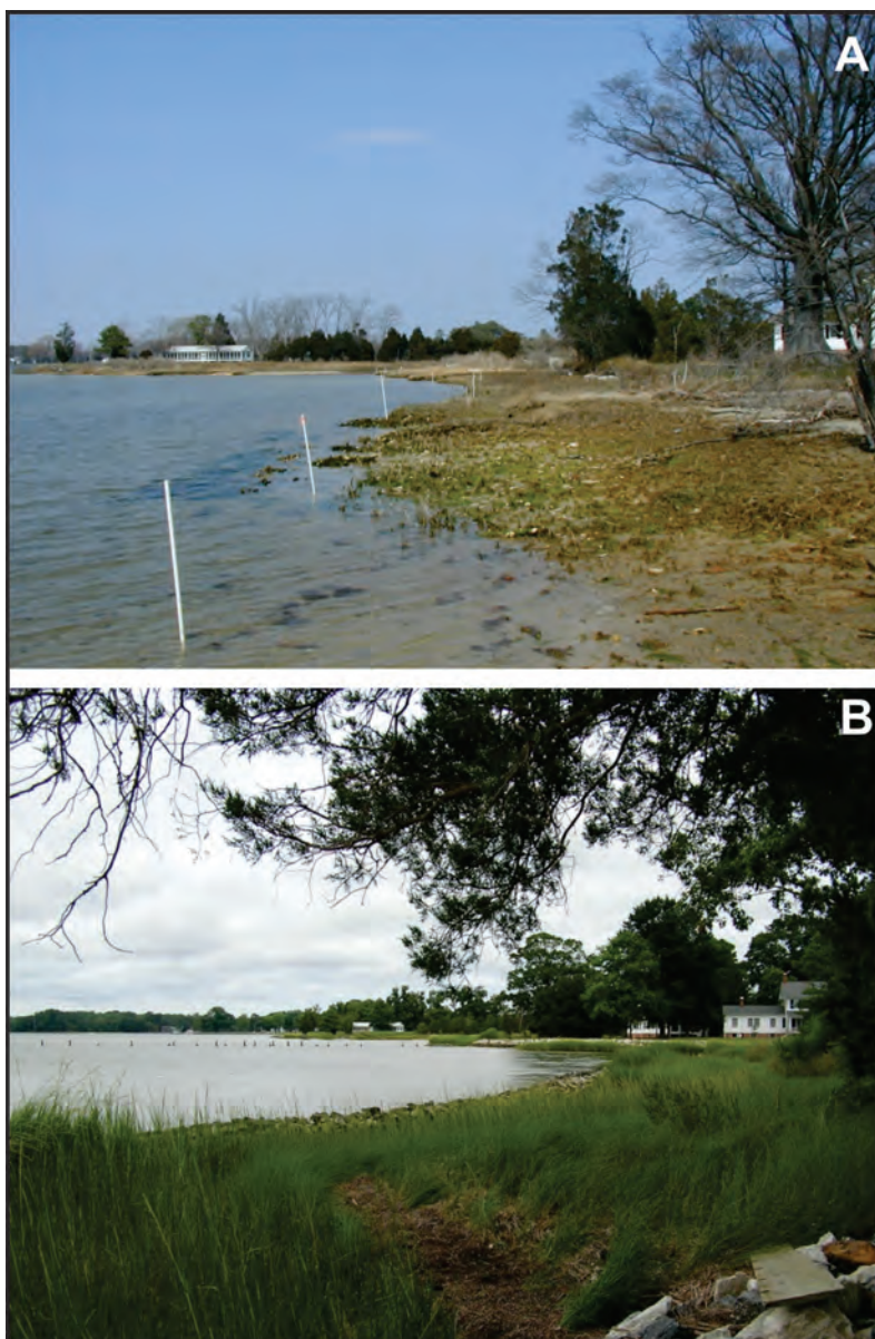
Figure 4-2. Hollerith marsh toe revetment/sill site A) before project with eroding fringing marsh in winter and B) after construction.
