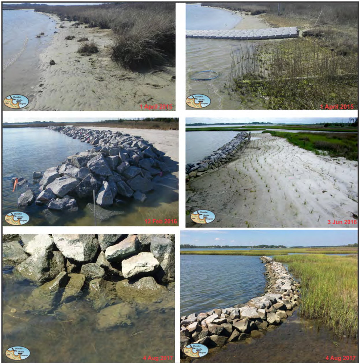
Figure 5-10. Captain Sinclair's Recreational Area pre-construction (top), post-construction (middle), and a year later (bottom). The marsh grasses are lush, SAV has grown behind the structure, and fauna are utilizing the rocks and the marsh.
