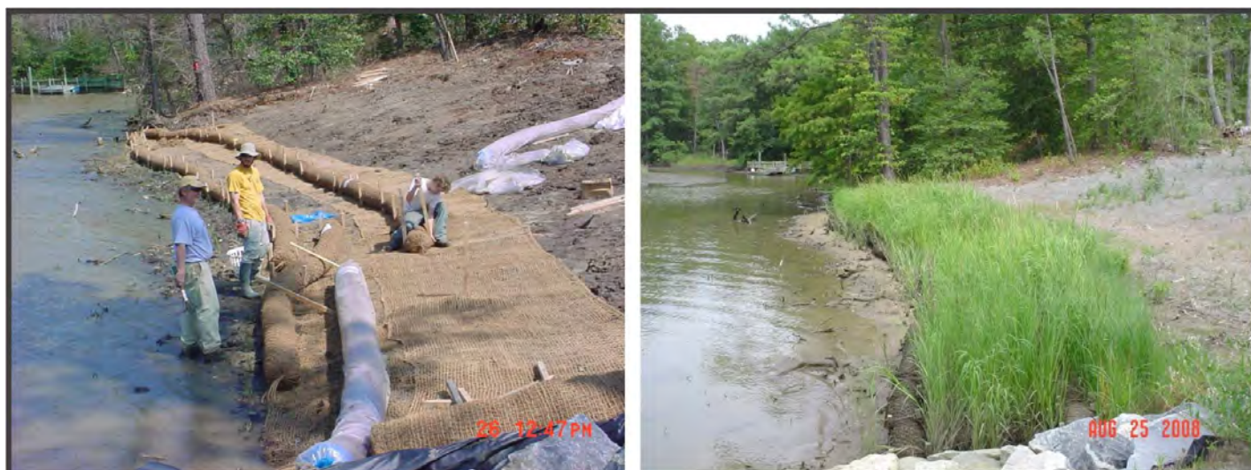
Figure 3-2. Coir logs and mats placed at toe of a graded bank for temporary stabilization while planted tidal marsh and riparian buffer become established. Photos by P. Menichino.
