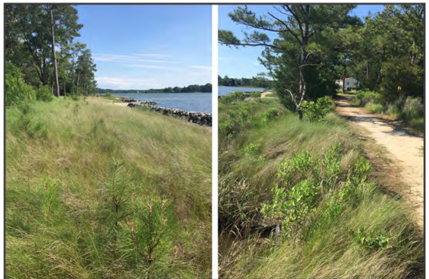
Figure 5-7. Photos of the project three years after installation in May 2017. The marsh behind the sill is expansive (left) and the access road is no longer threatened (right).
