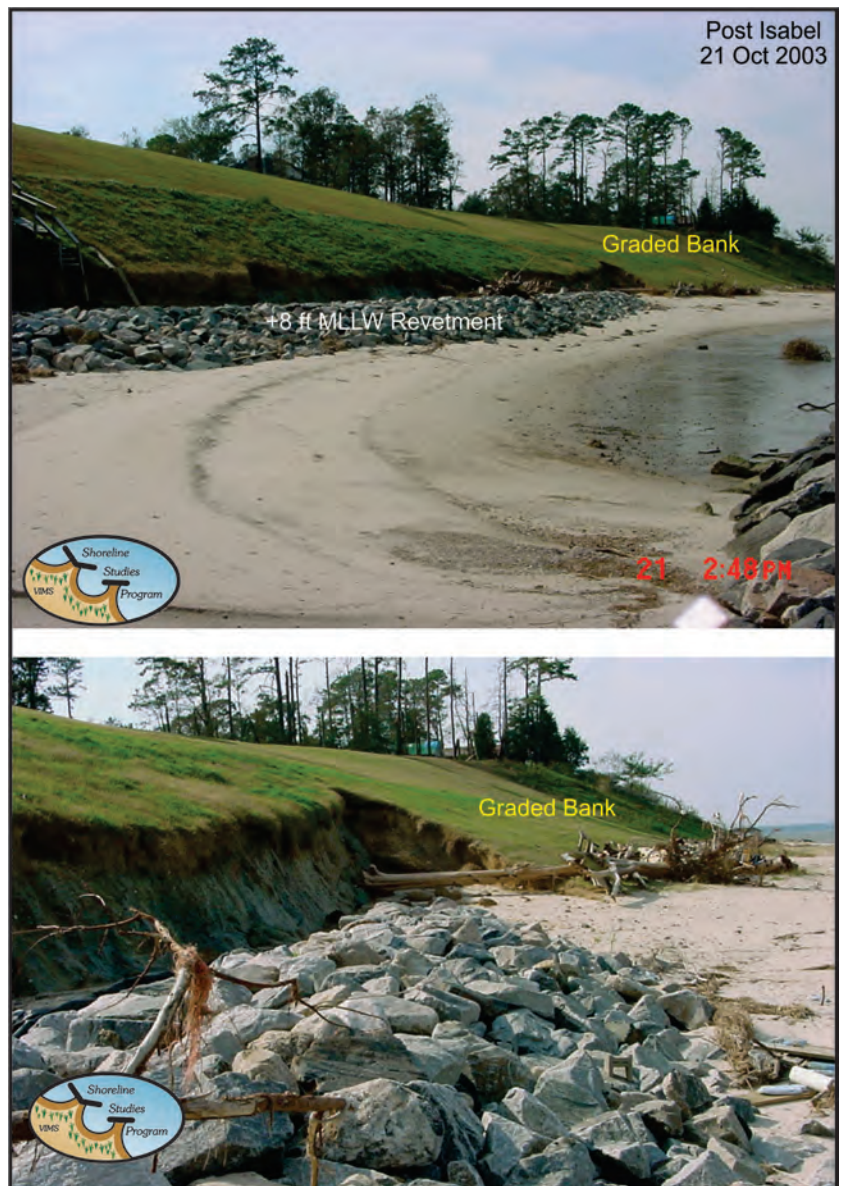
Figure 3-9. Revetment on the James River that was overtopped by storm surge and waves during Hurricane Isabel. Photo dates 21 October 2003.
