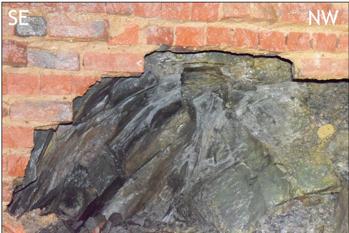
Figure 20. The low angle shear zone from the western portal that has been exposed from recent brickfall, and the area where sample WP-10 was collected.
