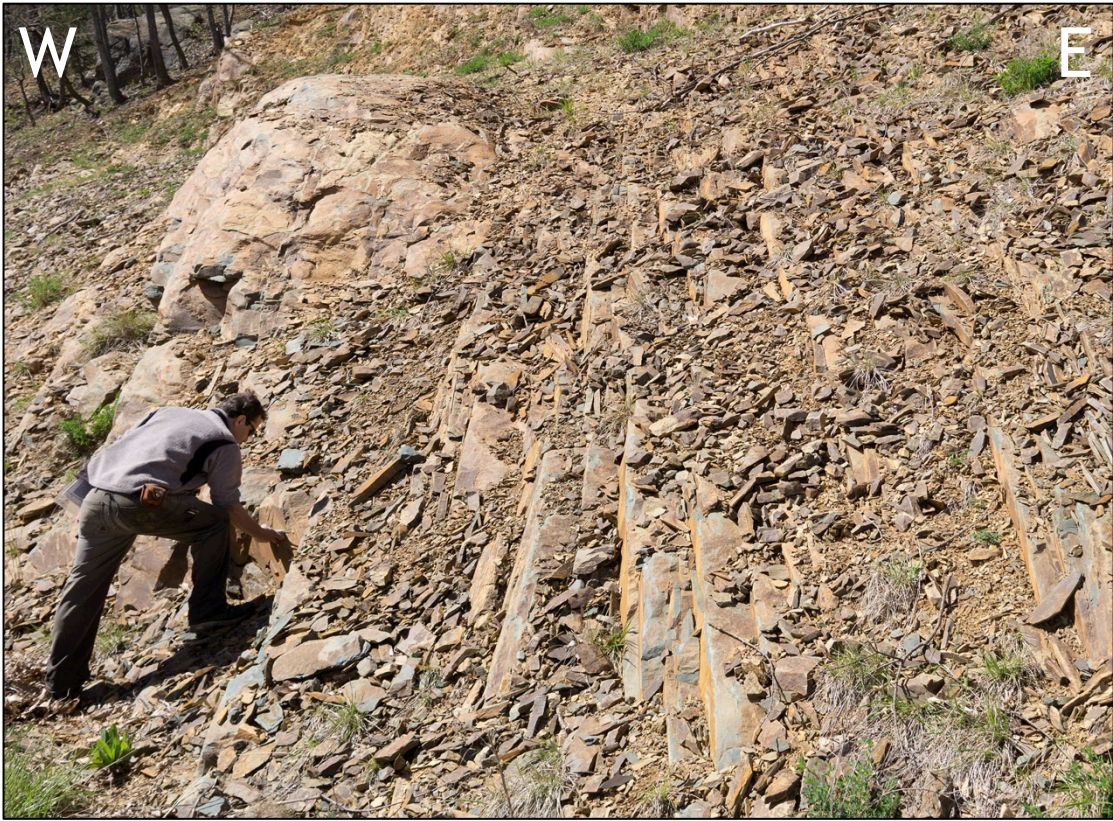
Figure 32. The high density fracture zone near the eastern portal entrance of the Blue Ridge Tunnel, with a majority of the fractures striking to the NW. The greenstones here are highly weathered, hence the tan to red color.
