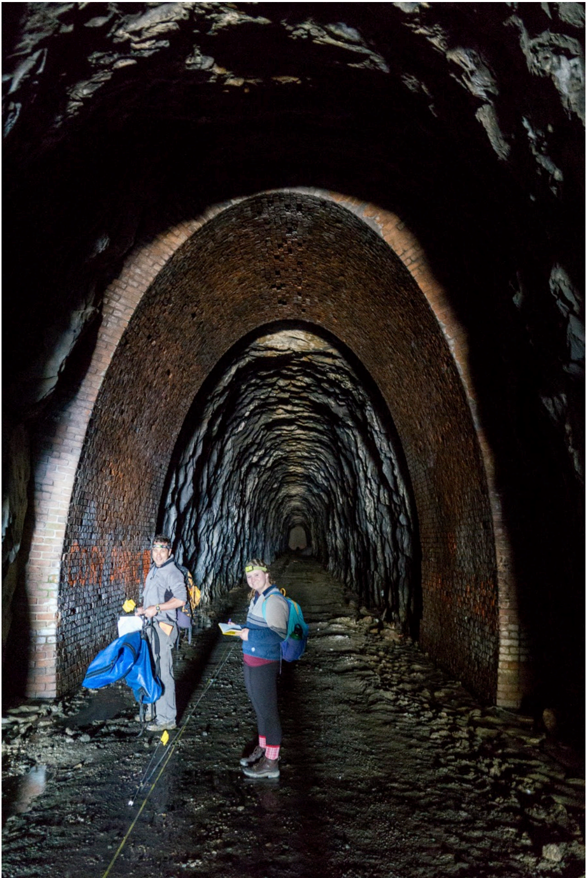
Figure 44. The probable test arch from the eastern side of the Blue Ridge Tunnel.
