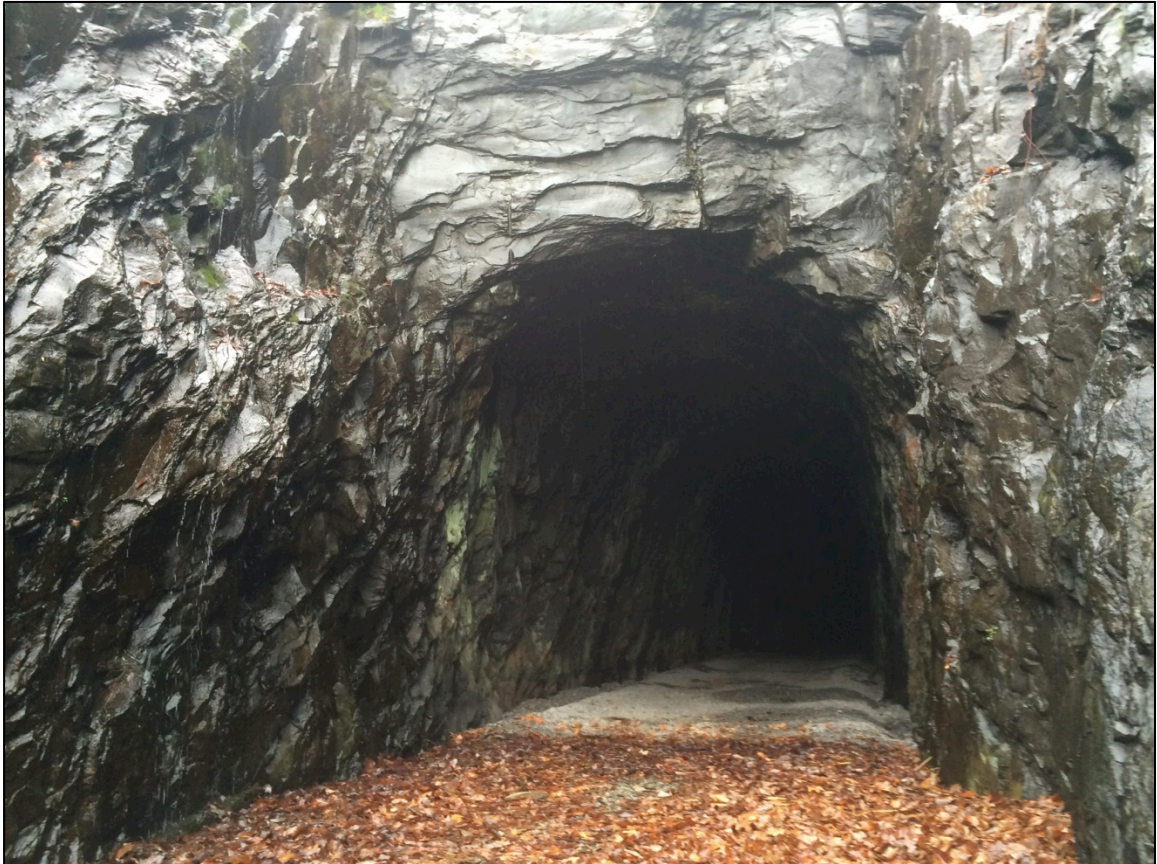
Figure 43. The eastern portal entrance is cut directly into the Catoctin metabasalt bedrock and has little to no evidence of rockfall or structural instability. Note that the tunnel has a roughly elliptical shape, which has lent itself to remaining intact for about 160 years.
