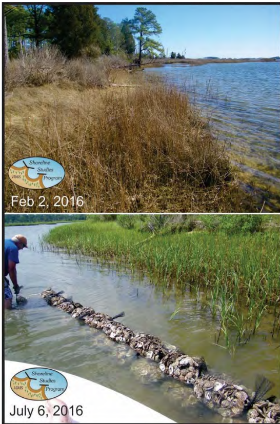
Figure 4-25. Site 6 Top: prior to installation, the site had an eroding marsh. Bottom: a 3-bag oyster bag sill was installed in July 2016.
