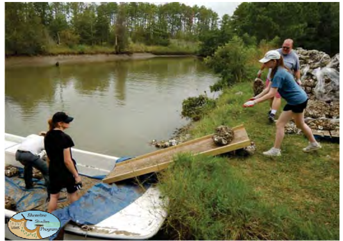
Lack of access at the site of placement meant that the bags had to be transported by boat. Because a 5 ft bank occurred at the staging area, a wooden ramp was built so the bags could slide down.
