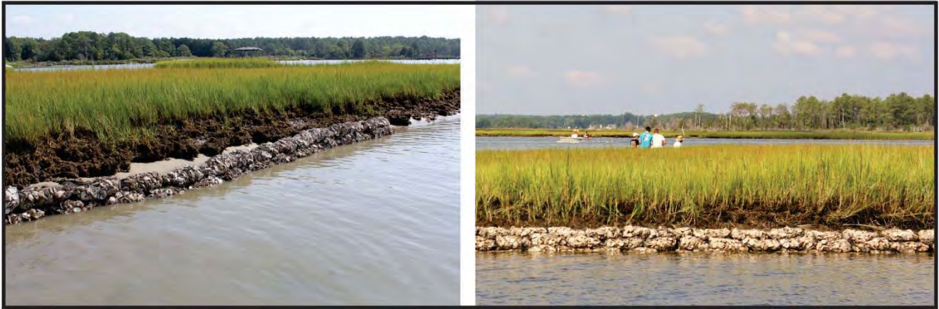
Figure 5-7. Construction of the 3-bag sill (left) and 6-bag sill (right). Photo credit: Linda Tjossem.
