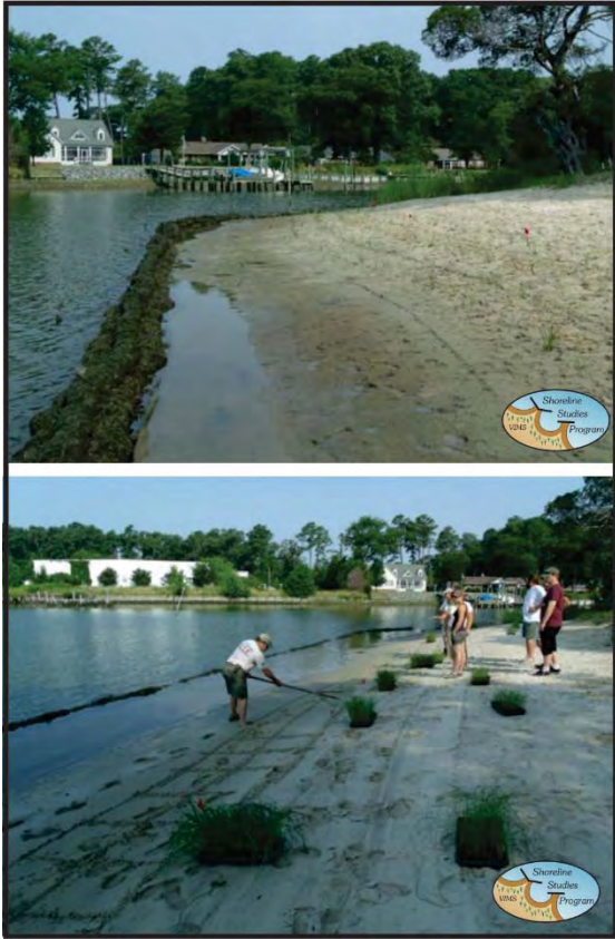
Figure 4-5. Post bag and sand installation at Site 1. The sand fill is visible landward of the sill, and volunteers planted grasses on the fill. Photo credit: Walter Priest, 29 June 2011.
