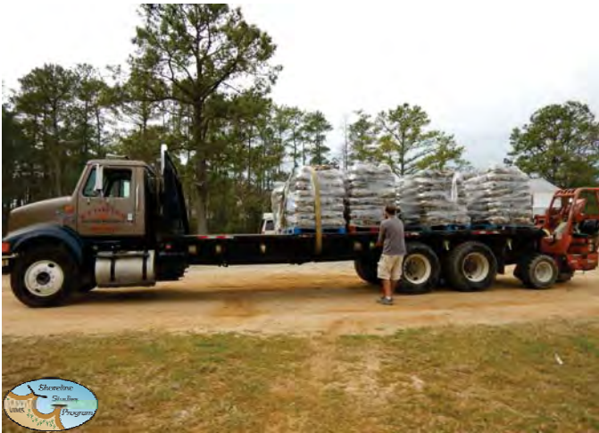
Oyster bag sills were delivered to the site by truck on pallets.
