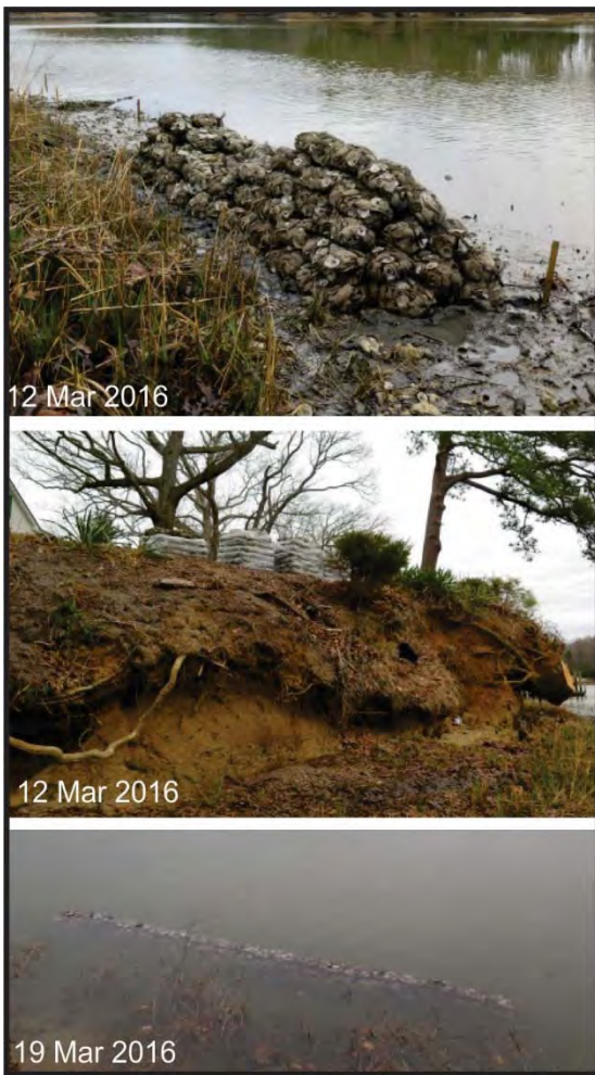
Figure 4-21. Site 5 during construction. Top: the bags are stacked in a 15 bag triangle at low water. Middle: the eroding upland bank was not graded. Bottom: the sill under high water. Photo credit: VMRC permit application.
