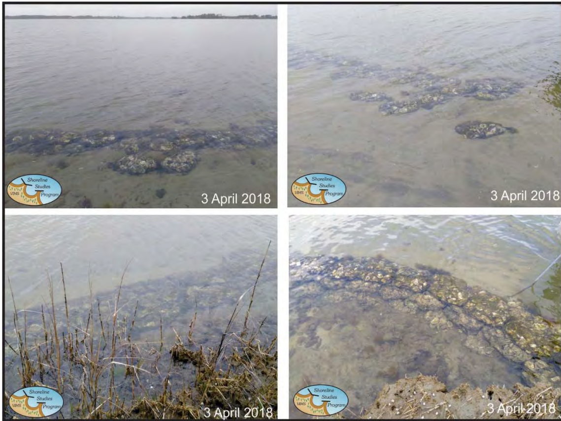
Figure 5-9. The three bag sill (top) that was placed on the southwest-facing shoreline has not been as stable. The top bag of some sections were rolled toward the shoreline. The six bag sill (bottom) on the point and the southeast-facing shoreline has remained intact.
