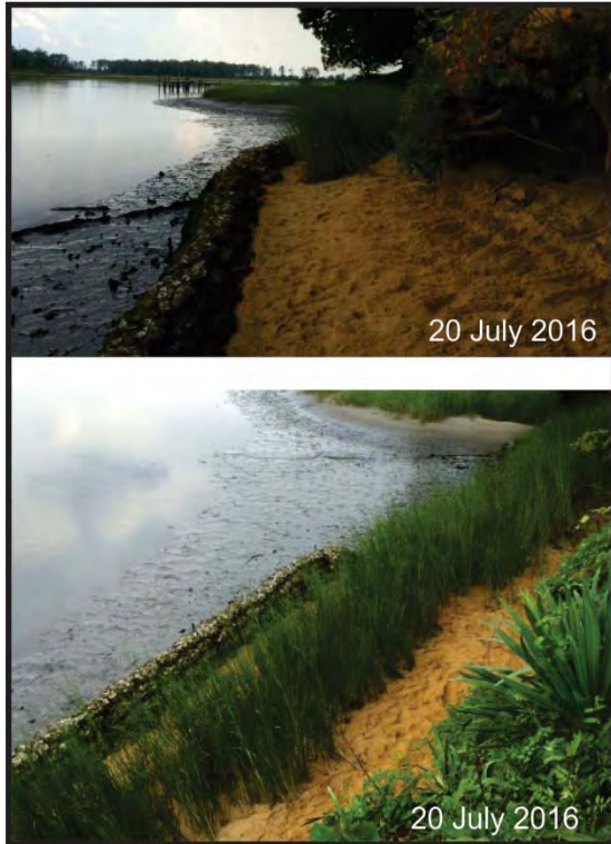
Figure 4-23. Site 5 during construction. Top: Sand was placed along the shoreline. Bottom: Marsh grass was planted. Photo credit: VMRC permit application.
