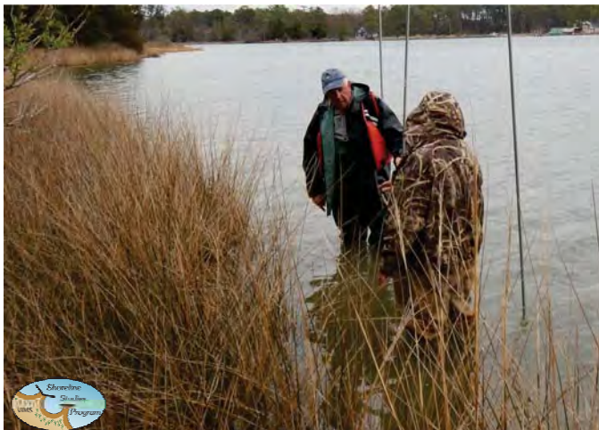
Metal pipe was installed to lay out the locations for the sills.
