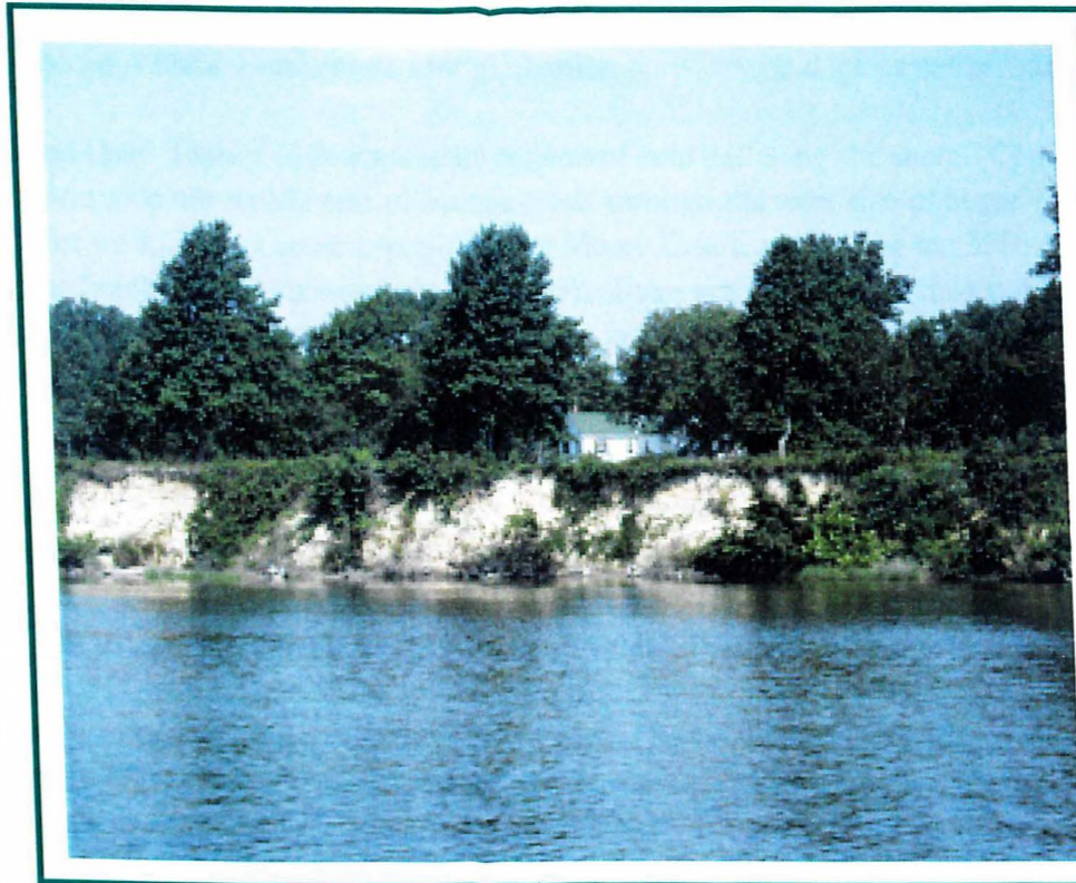
Eroding banks outside Cores Creek in Middlesex County
