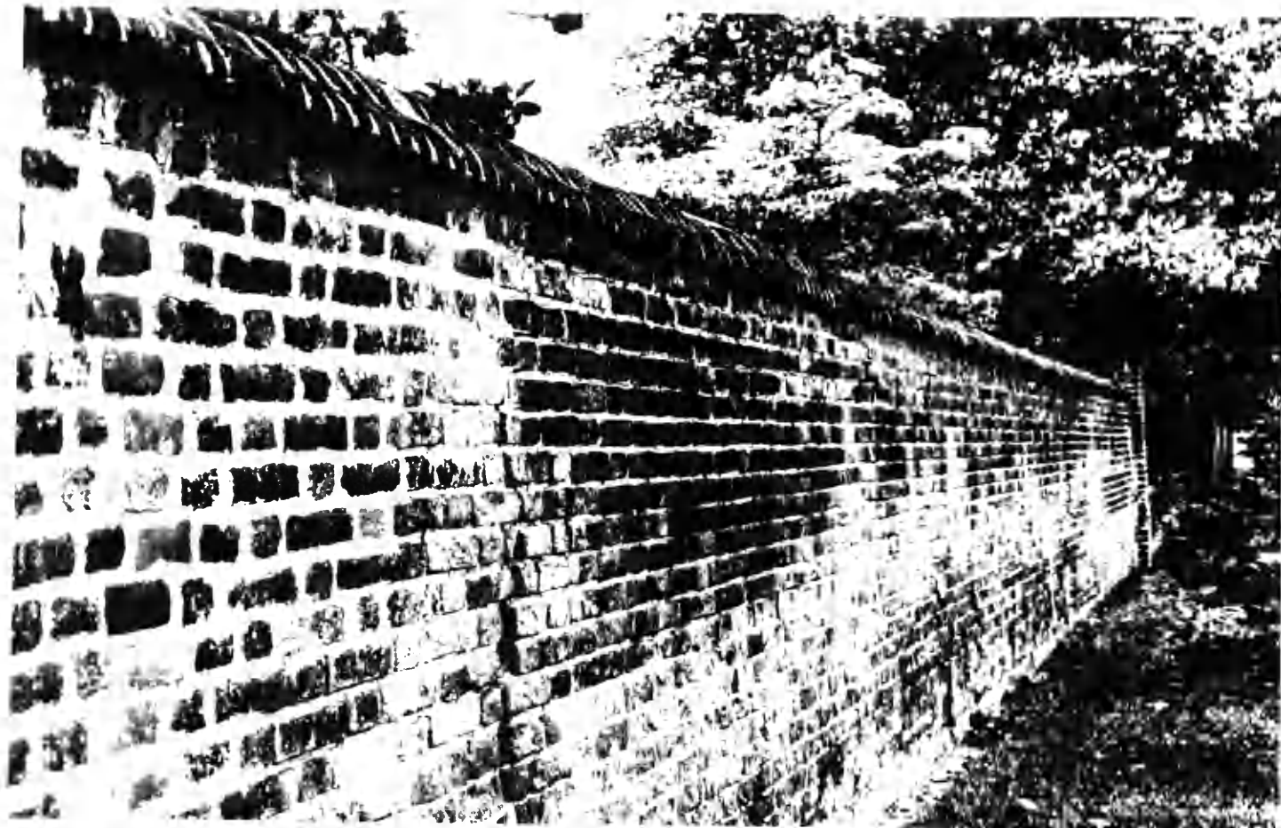
Plate 25 A portion of St. Paul's Churchyard wall as it stands in 1982; The walls are much repaired with a mixture of bonds.
