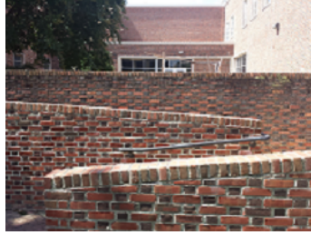
Figure 2.11: This figure shows a picture of three the wall that form the sides of the wheel chair ramp
