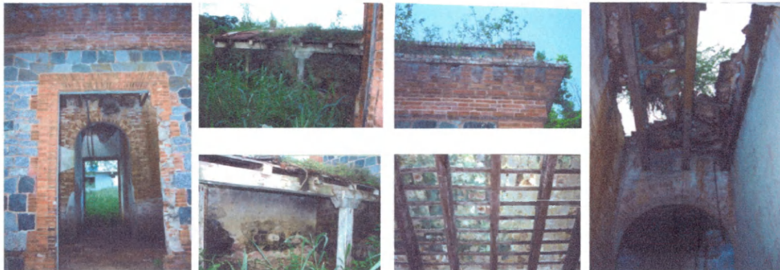
Photos 23-28. Details: central hall, zinc-covered shed, cornice, ceiling, roof construction. Model #3a casilla , Aibonito.
