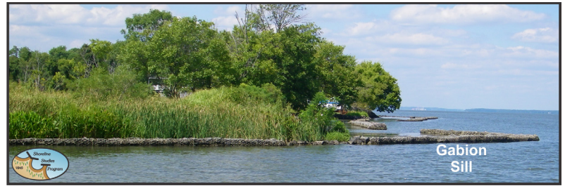
Figure 2-7. Reach 2, at the mouth of Potomac Creek, a gabion sill that has protected the shoreline for 20 years.
