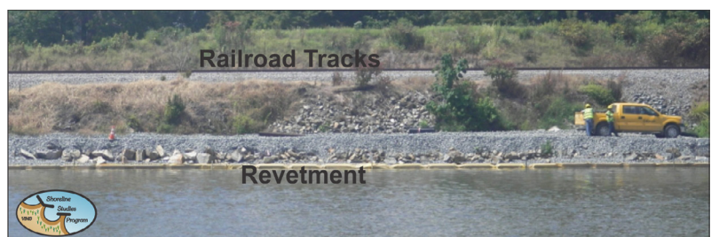
Figure 2-17. Reach 5, construction of a new revetment along the Potomac River that will protect the eroding shoreline that is very close to railroad tracks which are still used daily to carry passengers and freight.
