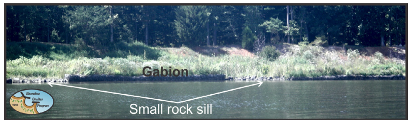
Figure 2-15. Reach 5, gabions along the shoreline that are providing effective shore protection along the Potomac River.
