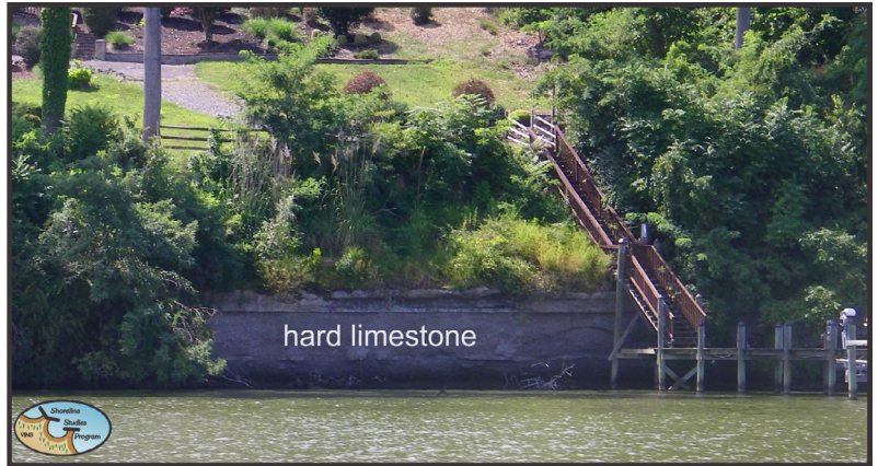
Figure 2-8. Reach 3, Potomac River high bank shoreline with a hard, erosion resistant limestone base of bank.
