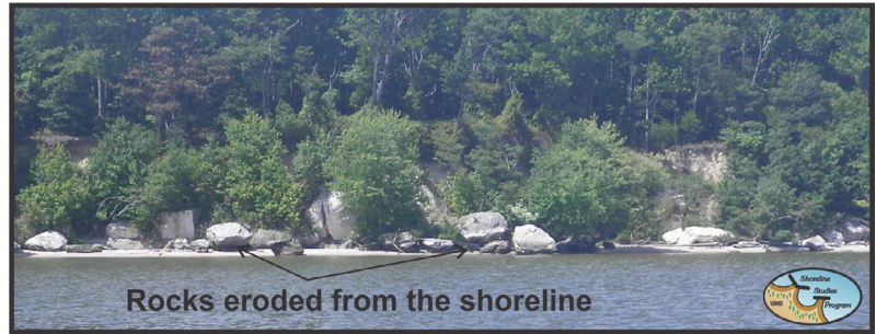
Figure 2-18. Reach 5, very hard rocks that have broken off from the bank along the Potomac River shoreline
