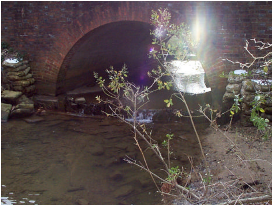
Figure 2. Brackens Pond spillway and tailrace. Irish ramp was set against the right wall on upstream end of culvert.
