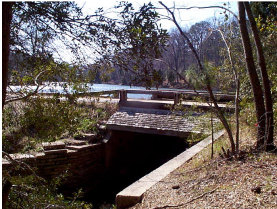
Figure 3. Bridge over Wormley Creek with Wormley Pond in background. Irish ramp was set under upstream edge of bridge at the base of the dam.
