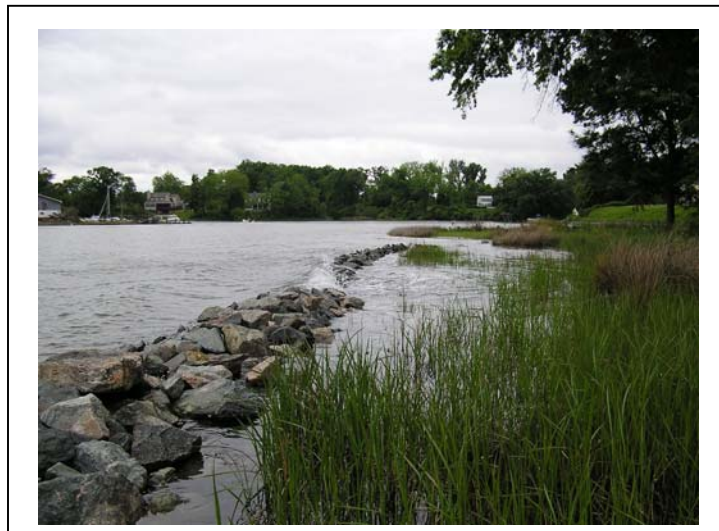
Figure 2. Boat wakes were observed washing over this marsh toe protection structure located in close proximity to a navigation channel. Boat wakes influence the wave climate in low energy settings.
