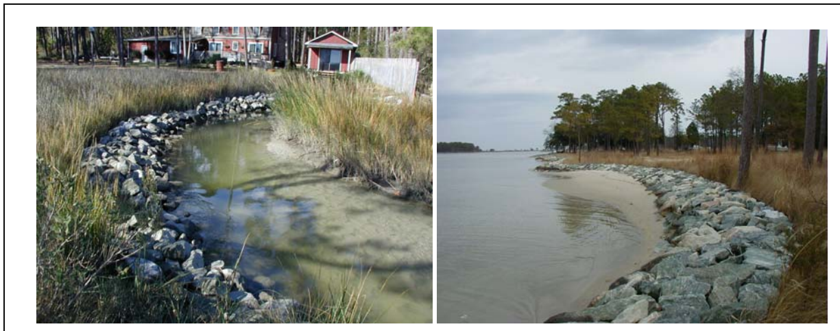
Figure 5. Unnecessary and inappropriate applications of marsh revetments are illustrated with these examples. The project on the left was located in a tidal channel and is excessive and unnecessary for erosion control (MA03). The project on the right was designed to perform like an upland revetment (LA07).
