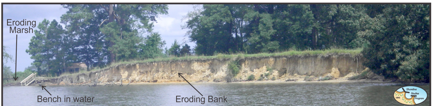
Figure 5-4. Eroding shoreline at Area of Interest 1 on Purtan Bay.
