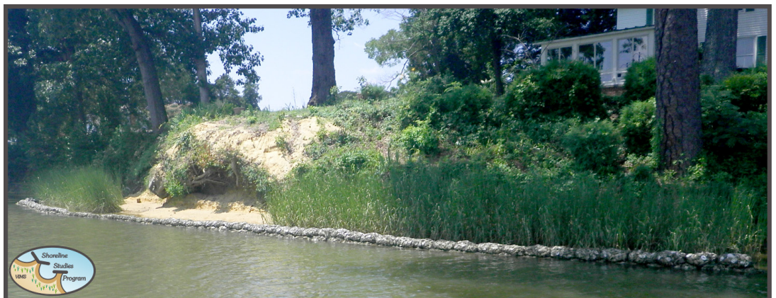
Figure 2-11. Eroding upland banks protected with a recently-installed oyster bag sill.
