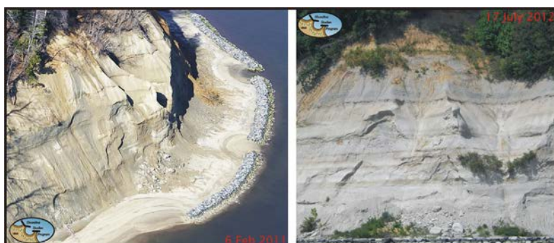
Figure 3-7. High sills built along the Potomac’s high energy, high bank shoreline. The material that slumps from the bank will be caught behind the sills and stabilize the base of the bank by protecting it from wave attack. A more recent photo shows that the slump material is starting to become vegetated.
