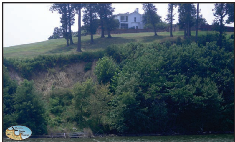
Figure 2-12. Along the Gunston Cove shoreline, the high upland bank is mostly in a natural state and is erosional.
