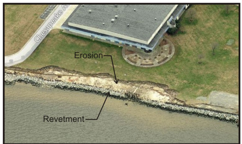
Figure 2-5. Bing map photo showing the rock revetment at Tidewater Community College and the erosion that has taken place landward due to overtopping during storms.
