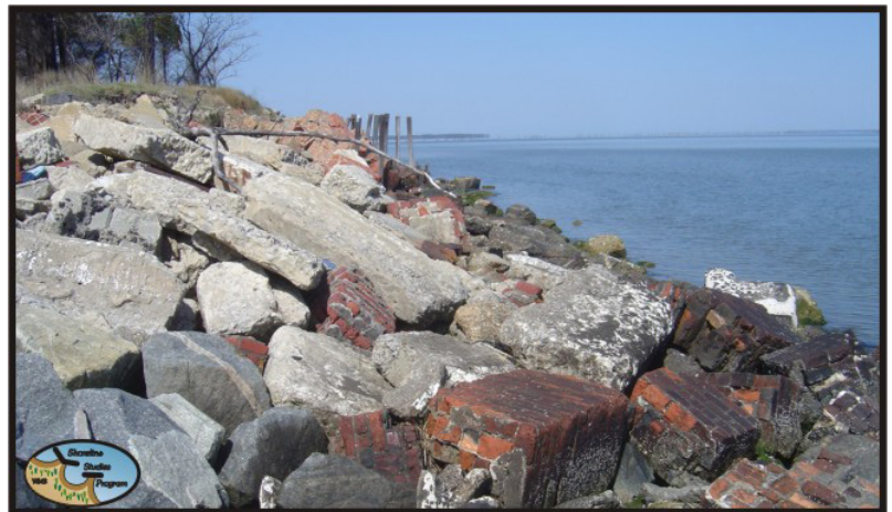
Figure 2-4. Broken concrete revetment along the James River shoreline east of the Nansemond River.
