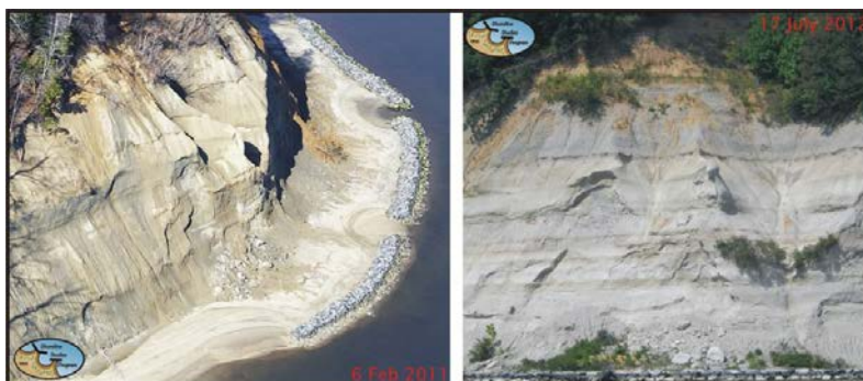
Figure 3-7. High sills built along Westmoreland State Park's high energy, high bank shoreline. The material that slumps from the bank will be caught behind the sills and stabilize the base of the bank by protecting it from wave attack. A more recent photo shows that the slump material is starting to become vegetated.
