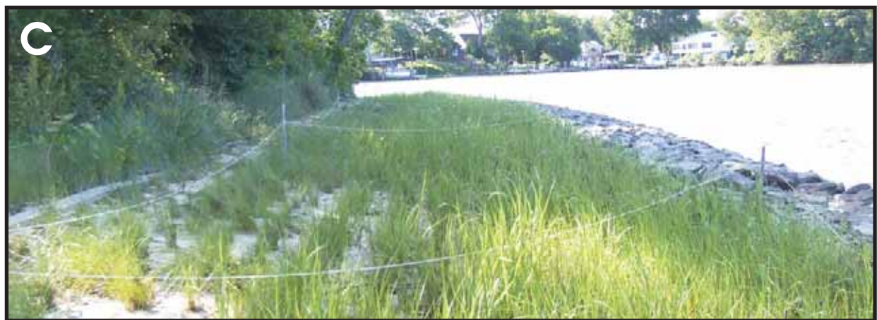
Figure 4-9. Hull Springs Farm shoreline A) before construction, B) after construction of the sill and placement of sand, and C) after planting.
