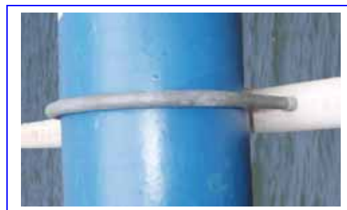
Figure 5.16 The guard-pipe is fastened to the transverse PVC by a U-bolt
