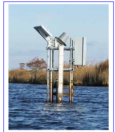
Figure 5.19 Galvanized structure. USGS monitoring station. (Source: Paul Perusse)
